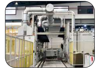
IPSEN Carburising Equipment (Germany-made)
